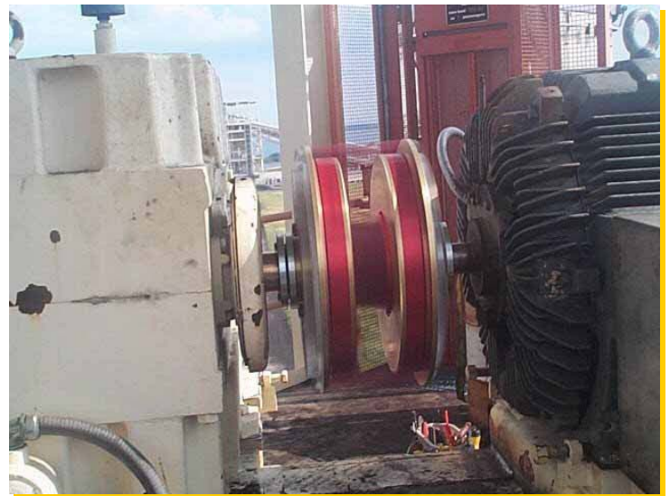
▲ MGTL 12/20, Power Generation, Conveyor System, TX, USA
