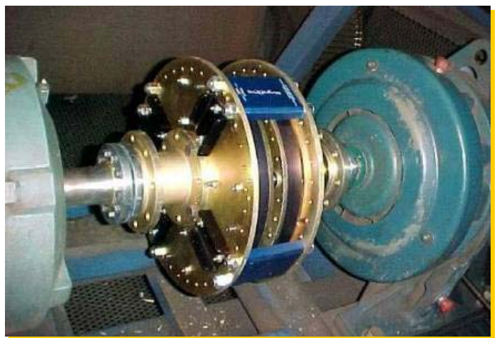
▲ MGD 14/40, 40HP, 1800RPM, Airport Conveyor System TN, USA
