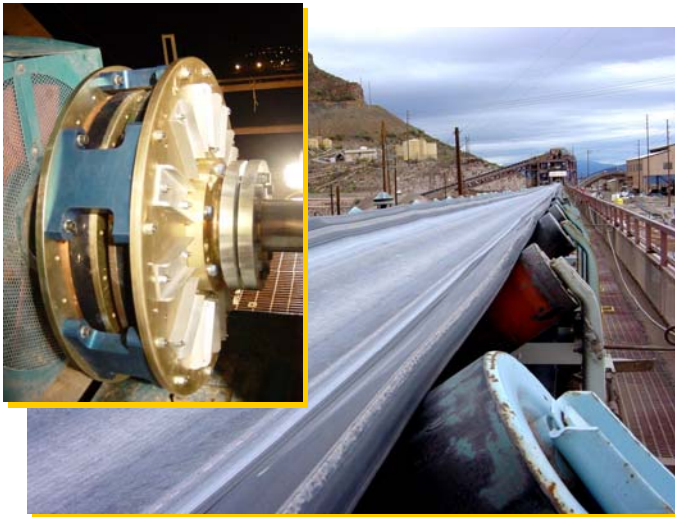
▲ MGD 20/400, 300HP, 1800RPM, Mining, Gear Box in Bulk Conveyor System, AZ, USA
