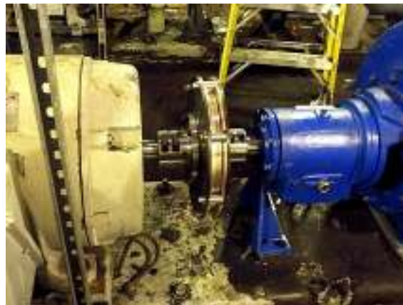
MGE-15, 150HP, 1800RPM, Power Plant, Pump – Lime Slurry Scrubber, Becker, MN
