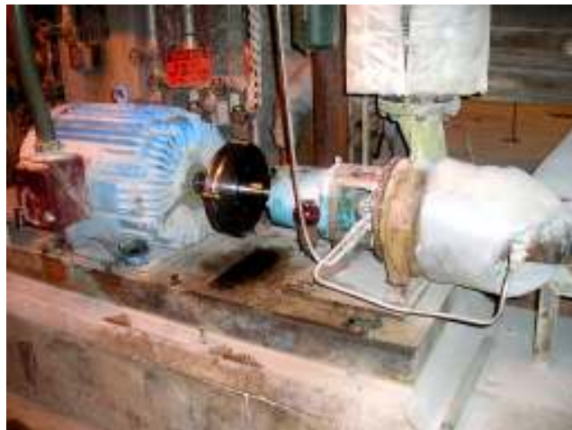
MGE-11, 100HP, 3600RPM, Pulp & Paper Plant, Clean Condensate Pump, St. Helens, OR
