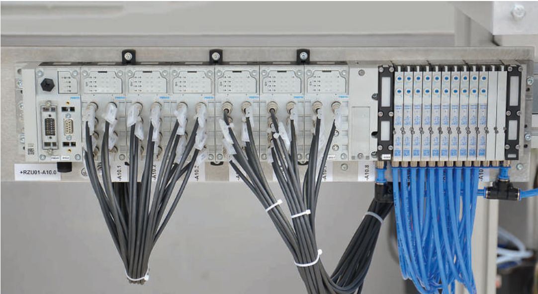
Valve terminal with input and output module
