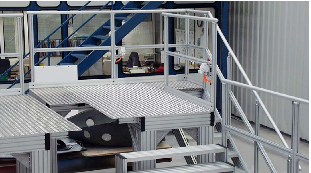
Platform with Series 40 hand rails along one side of platform and stairs
