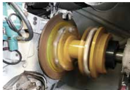
Torque monitoring on wind turbines.
